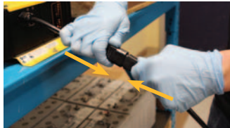
Figure 3: Reconnect AC power to the charger.
